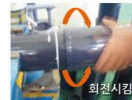
Quickly removing the fitting from the pipe after the first application of adhesive and rotation of the fitting 360° to insert it into the pipe up to the zero point
